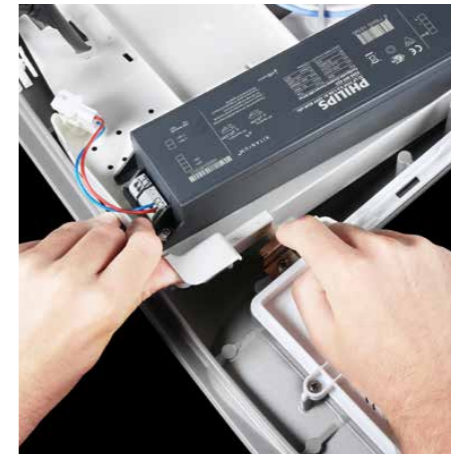
Removal of control gear.
